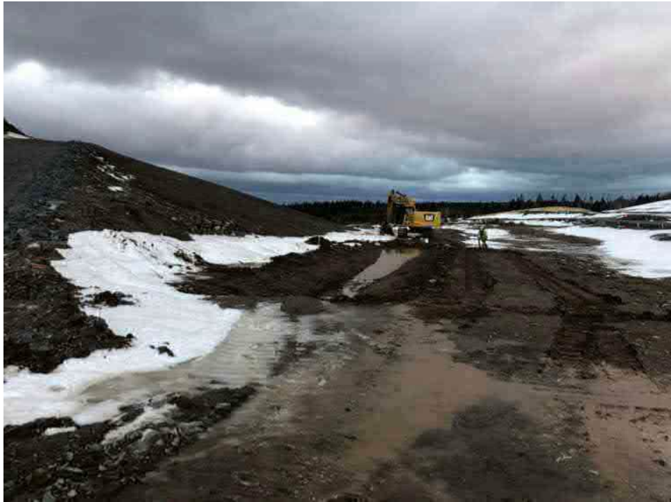
Photo 1: ARCP setting up pump to pump water out of the lined ditch excavation.
