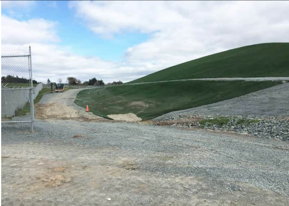
Photo 14: Eastern view of the north side of the main landfill cell area (capped) from the NW corner of the cell.
