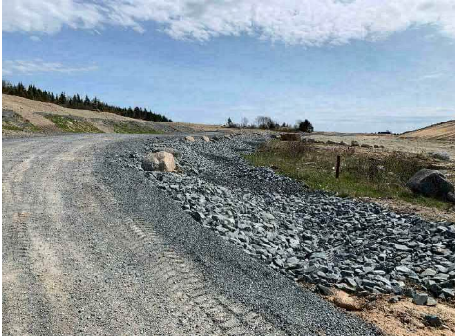
Photo 9: Rock lined ditch with rock and hay check dams. Ditch is located along the access roadway.
