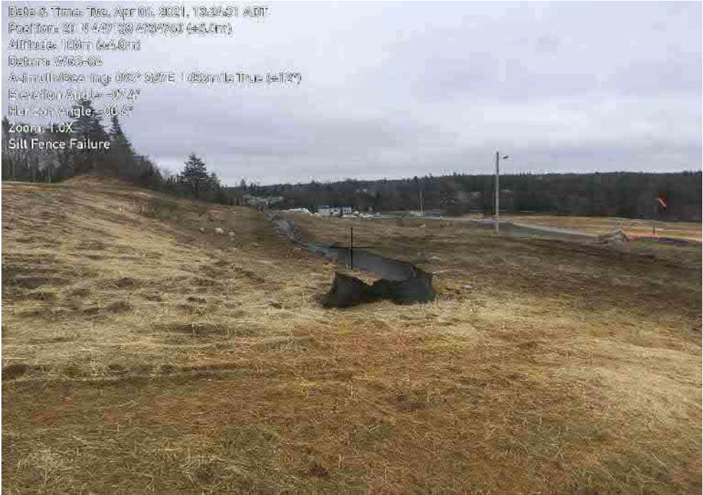
Photo 1: Silt fence failure south of existing fire pond. Corrective measures required.
