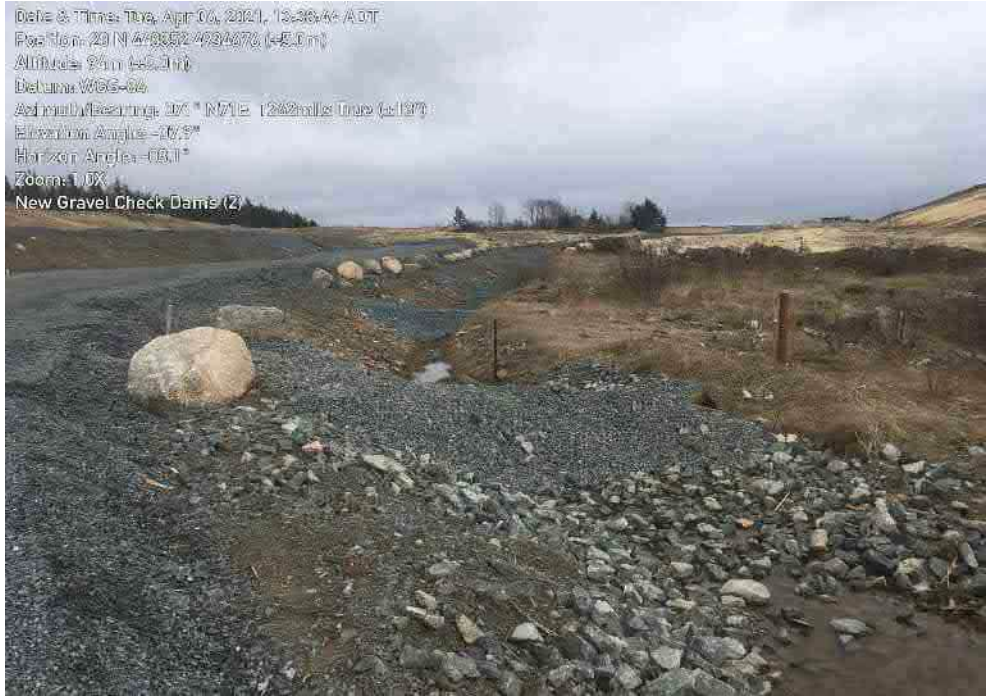
Photo 9: Installation of new rock check dams - retention of sediment upstream. Sediment presence indication of unstable surfaces upstream - Upstream areas require remedial action. Relatively clean water filtering through.
