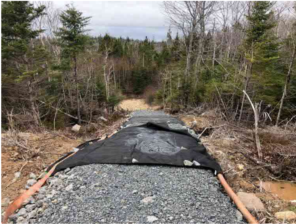
Photo 3: Pumps set up with silt bags if future pumping is required to control water during pending rain event(s).
