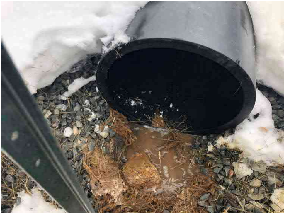
Photo 3: No discharge from the 500 mm discharge pipe once the blank was installed in the 150 mm ground water interceptor pipe.
