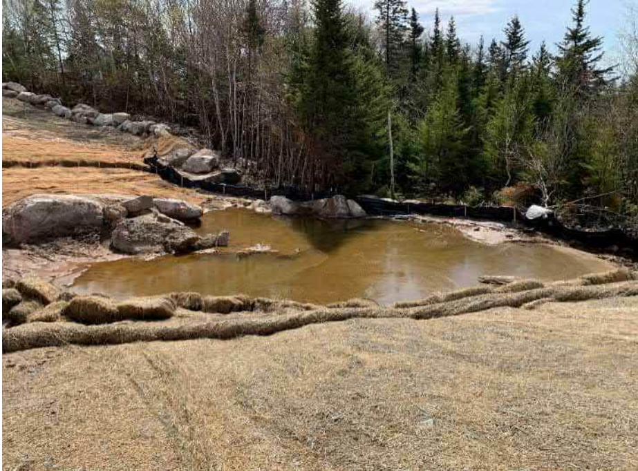
Photo 3: Basin at the bottom of former BDA ABO. Silt fencing, hay bails and cocomats placed surrounding the basin.
