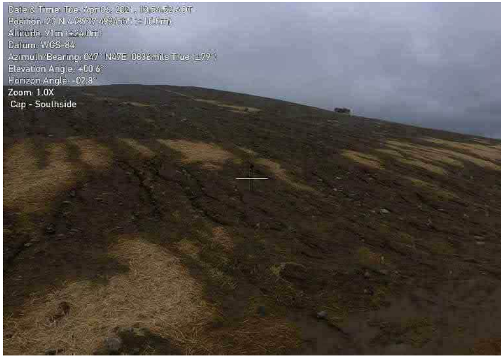
Photo 18: South slope of cell cap - erosion measure failure - immediate action required.
