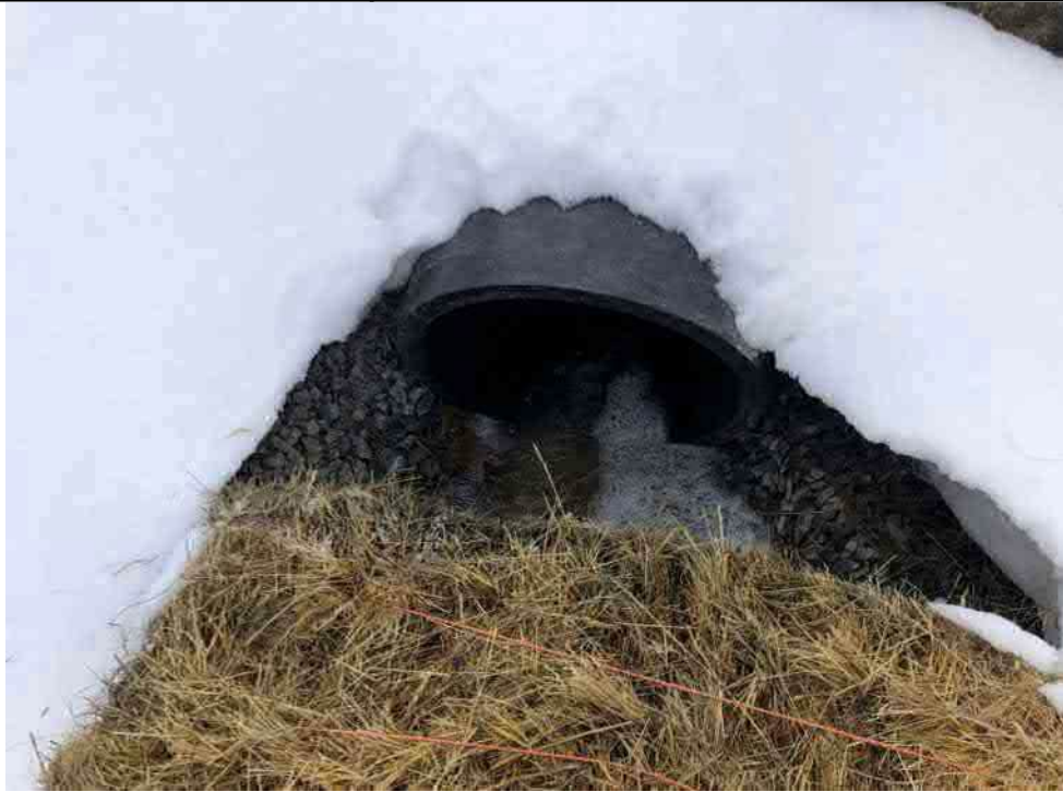
Photo 3: Flow from 500 mm discharge pipe prior to blank being placed in 150 mm pipe.
