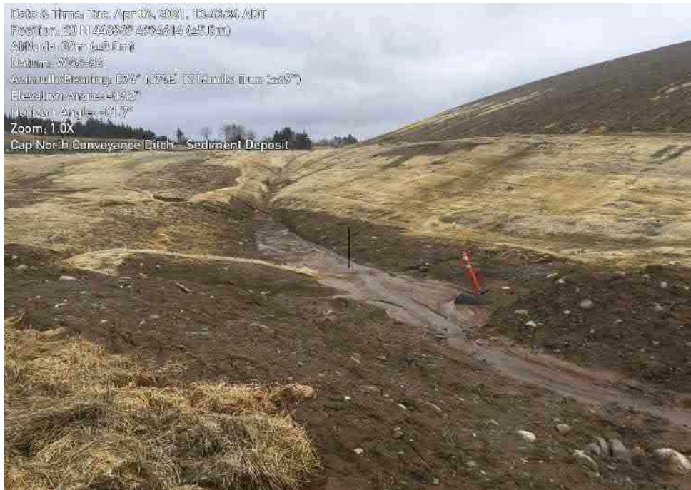
Photo 12: Swale on north side of cell cap experiencing heavy erosion and sediment deposit. Channel stabilization, rock check dams, and removal of sediment required. Storm sewer capped.
