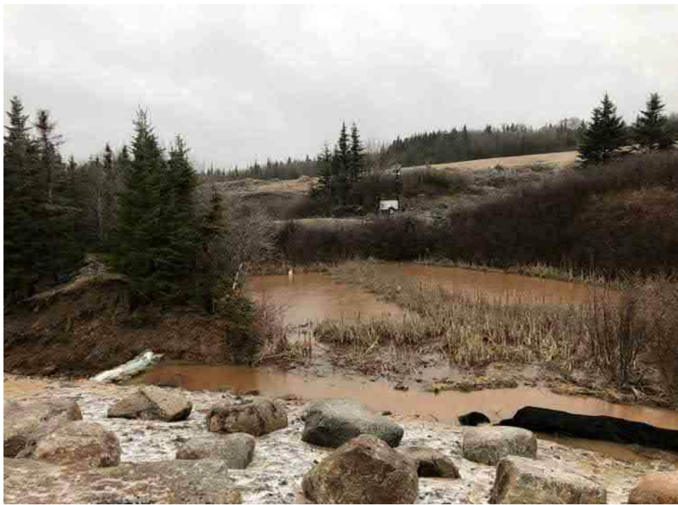
Photo 2: Silty water in settling pond, pumps setup to pump through filter bags (10:05am).
