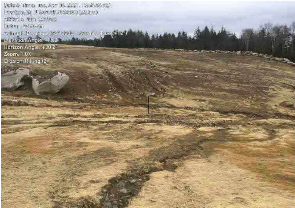
Photo 20: Southeast corner of landfill cap slope. Heavy erosion occurring. Re-grading and slope stabilization required, additional erosion control matting and biofilter check dams in localized channel. Immediate action required.
