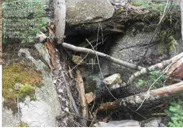
Photo 17: Berm corrected on existing pond - sediment laden water still short-curcuiting berm - immediate correction required.
