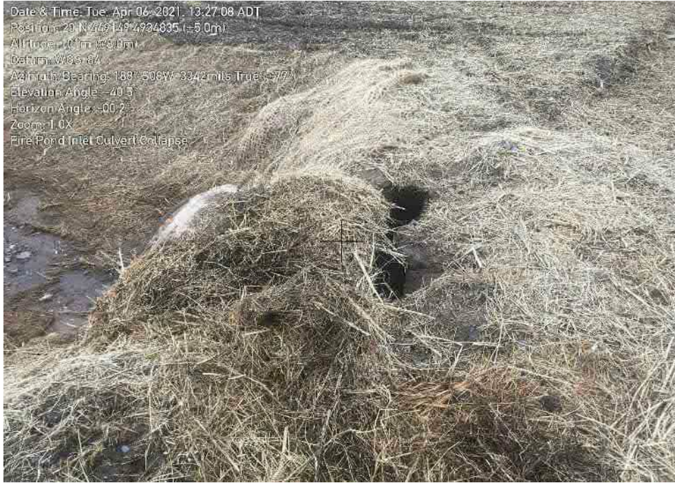
Photo 3: Culvert collapse/failure immediately upstream of existing fire pond. Corrective action required.
