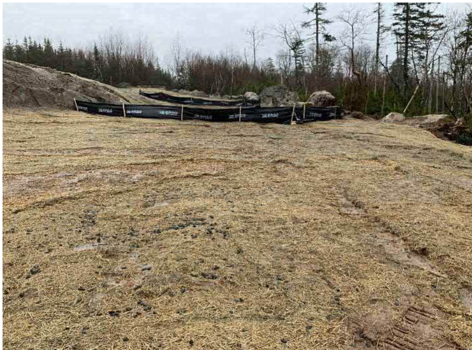
Photo 16: Three (3) silt fences placed across slope travelling to Sheas Lake.
