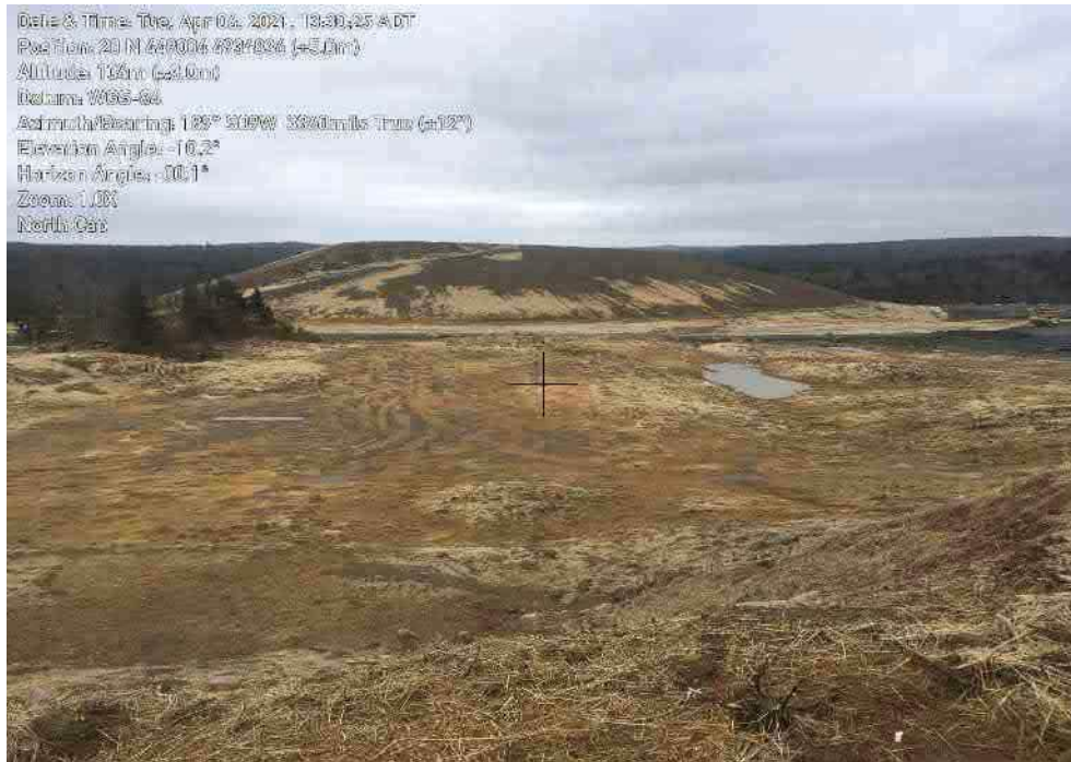
Photo 6: North-facing landfill cap - erosion measure failure - immediate action required.
