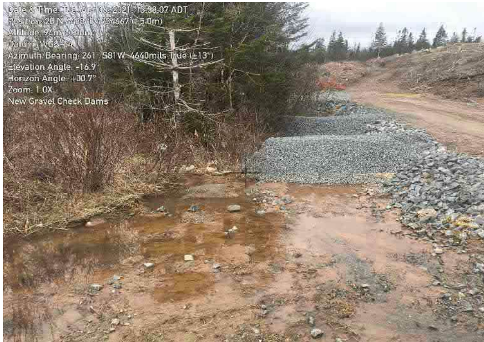
Photo 8: Installation of new rock check dams - retention of sediment upstream. Sediment presence indication of unstable surfaces upstream - Upstream areas require remedial action. Relatively clean water filtering through.
