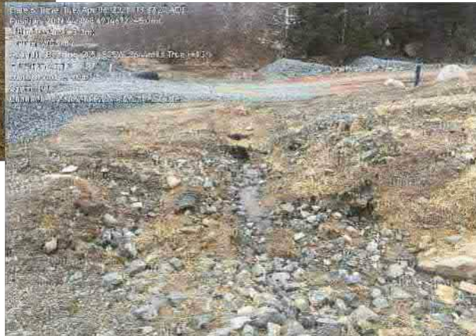
Photo 7: Erosion occurring in low-area west side of abandoned treatment pad. Culvert failure/crushed pipe exacerbating erosion.
