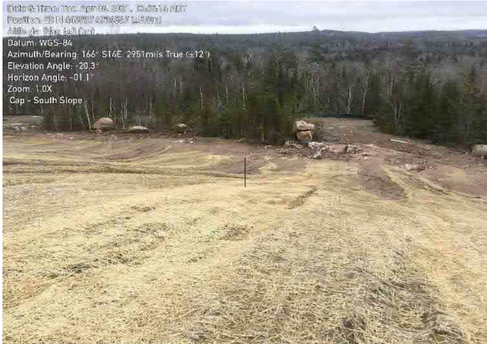
Photo 19: South slope of landfill cap - reasonable coverage of slope with erosion control mapping - incomplete in some areas with significant erosion present.
