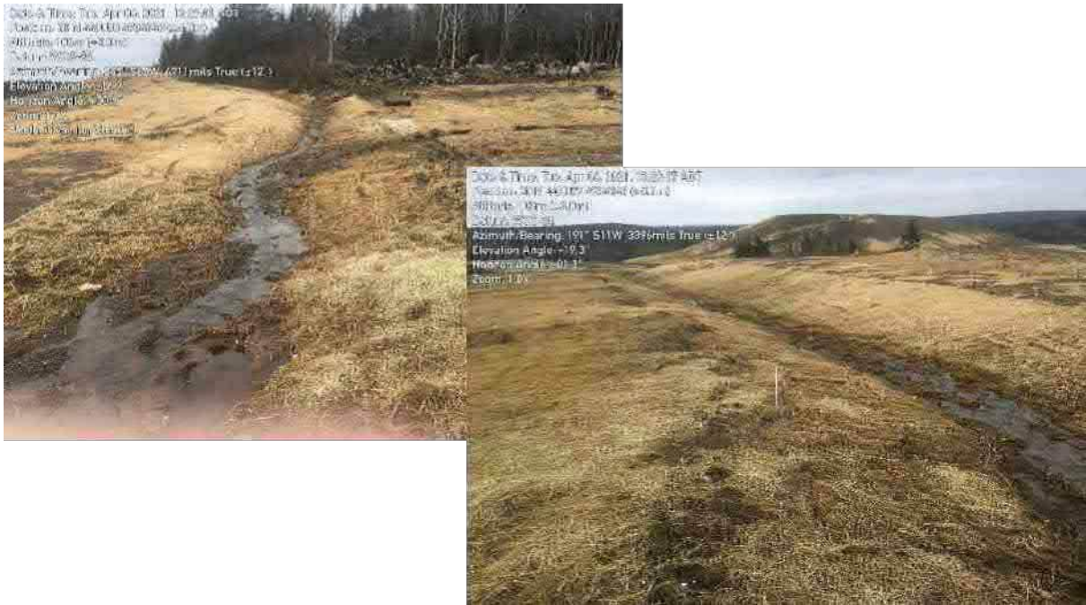
Photo 5: Easterly channel on north property line, erosion present, remedial action required, erosion control matting.
