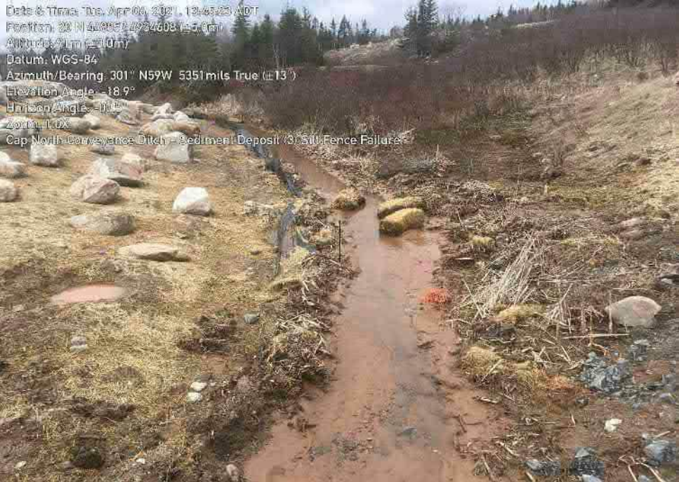
Photo 13: Channel with heavy sediment deposits, failed straw bale check dams and silt fence. Removal of sediment, stabilization of channel, and remediation of measures required.
