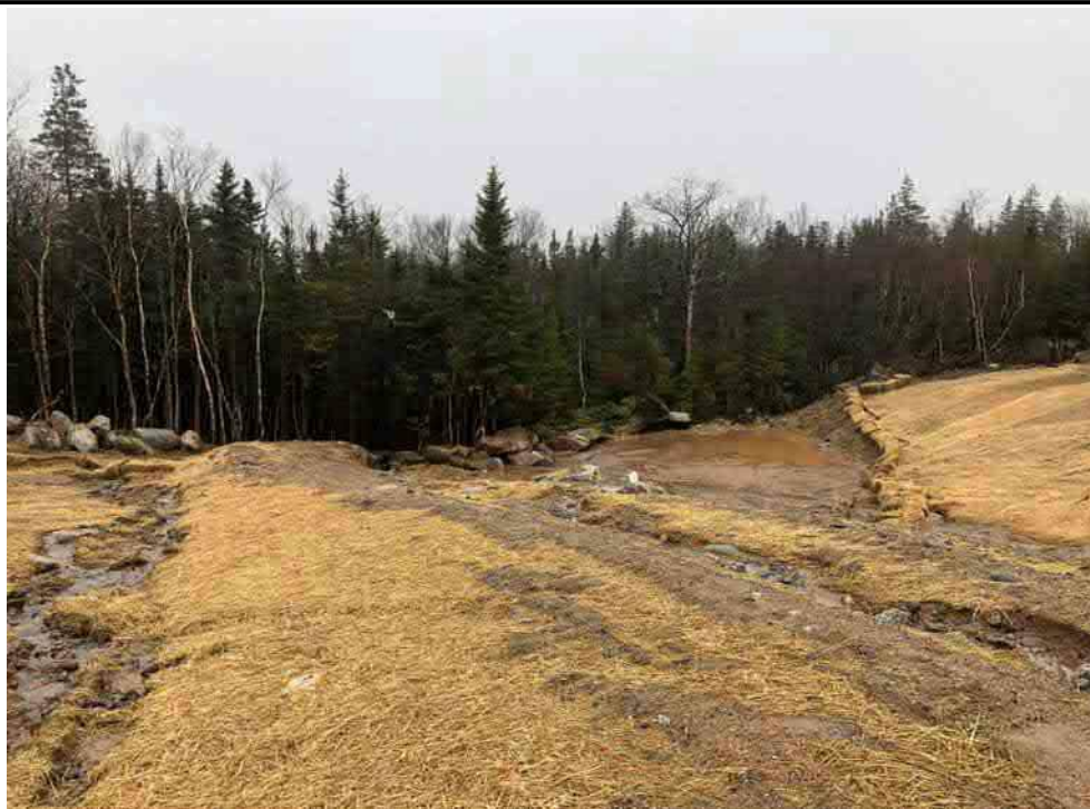
Photo 2: Erosion in BDA ABO.
