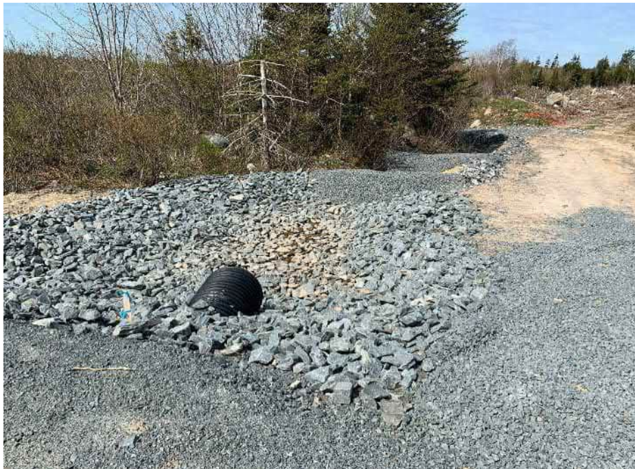
Photo 8: Rock lined ditch with rock and hay check dams. This flows into basin in Photo 5.
