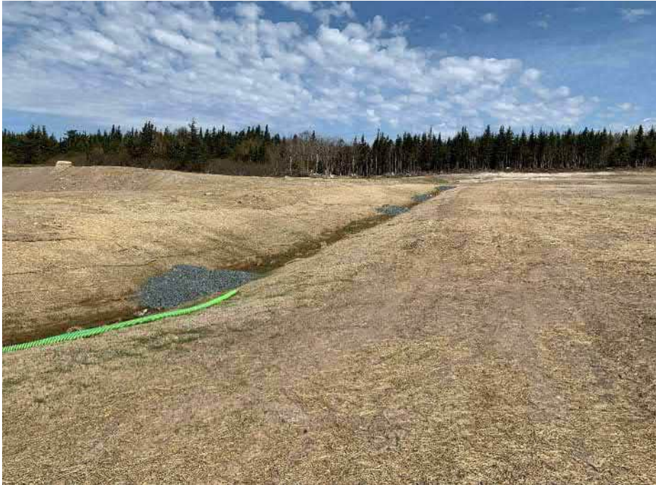
Photo 11: Cocomatting, hay bail and rock check dams placed in ditch dug through former BDA CDELM. The ditch travels from the North of the site to the access roadway ditching.
