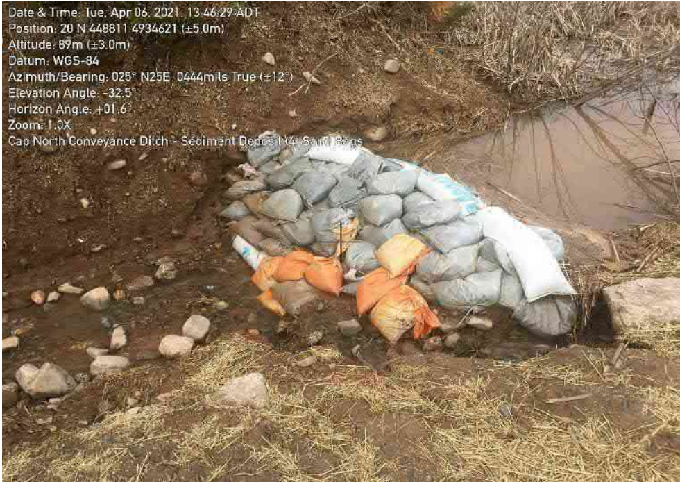
Photo 14: Sand bag check dam functioning well. Minor maintenance required to prevent short-circuiting along perimeter.
