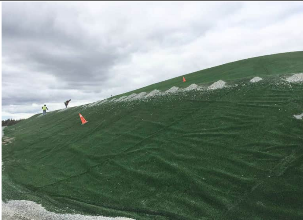
Photo 10: Western view of the south side of the main landfill cell area (capped) from the SE corner of the cell.
