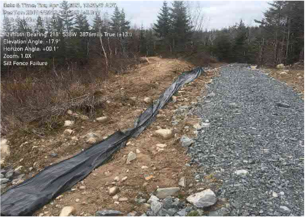
Photo 10: Silt fence failure south of existing fire pond. Corrective measures required.
