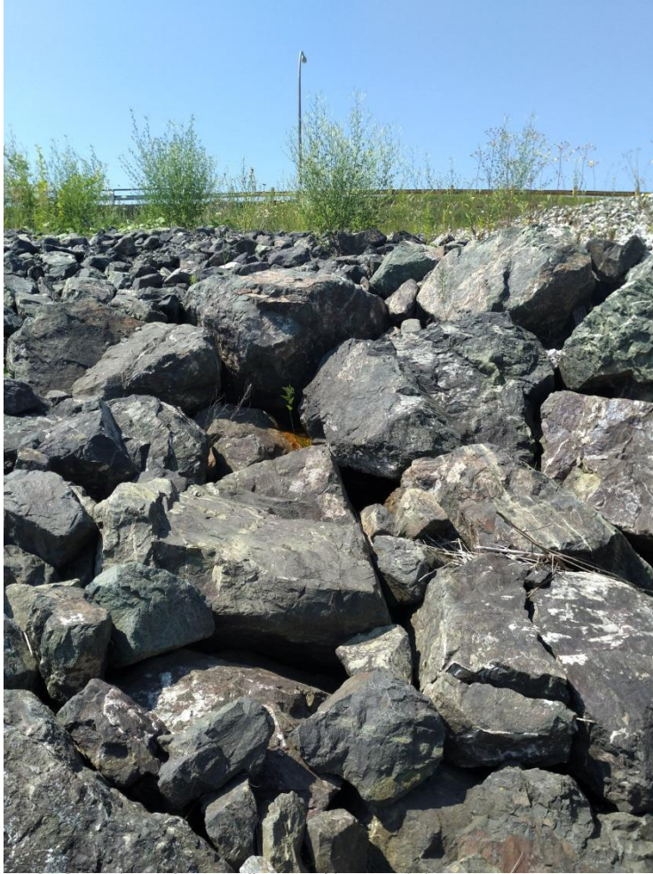
PHOTO 7: View of water flow and iron staining on Riprap south of COB-4-SW at looking south.
